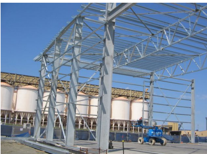
The steel supports for the 15,000m 2 cargo shed begin rising out of the Port Kembla site
