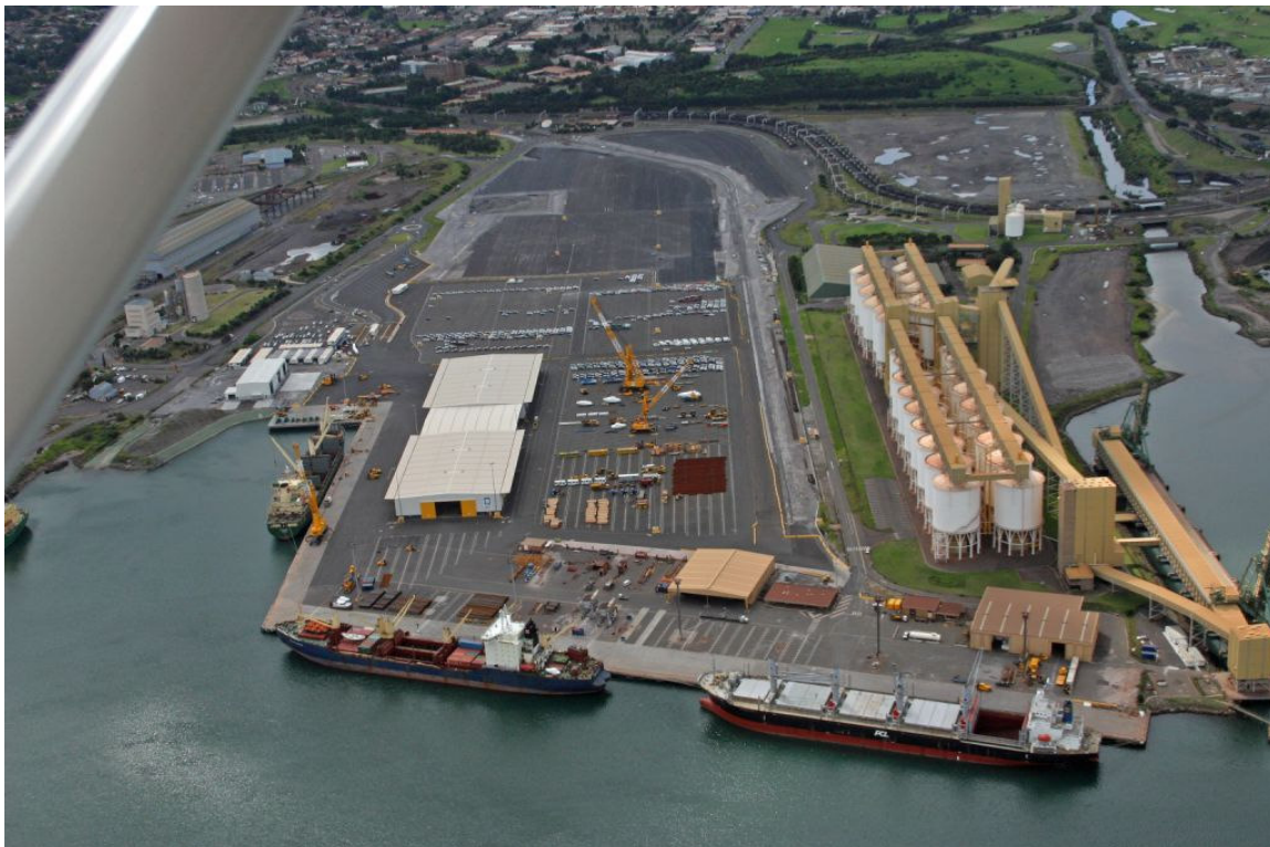
An aerial view of progress at the $80 million Port Kembla facilities showing the newly paved PDI area (at the top of the photo) nearing completion.
