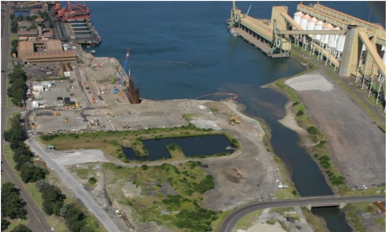
Construction works underway at the new berth 103 which will provide valuable additional facilities to support the main terminal site.
